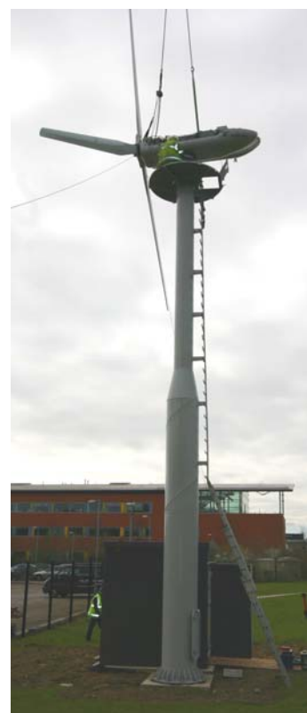
Figure 1: Photograph of the wind turbine as installed in Cambridge.
