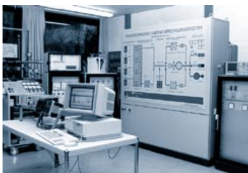
Control and communication laboratory
