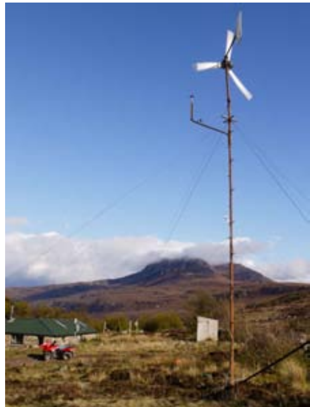
Figure 4: Data logging set up on the 3m diameter turbine.
